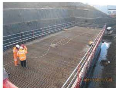
Attenuation Tank, Edinburgh Gateway
