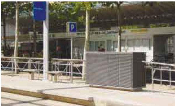
EQUIPMENT CABINET, MONTPELLIER
