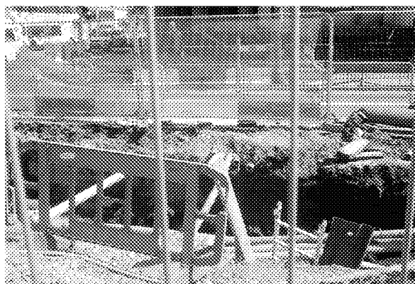
Photo showing shallow ducting
