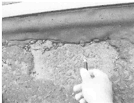
(This photo clearly indicates of thin the wearing course is at the location)
