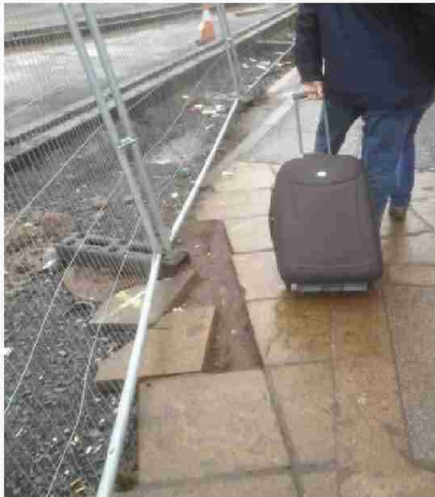
Broken paving slabs and trip hazard Outside Haymarket Station
