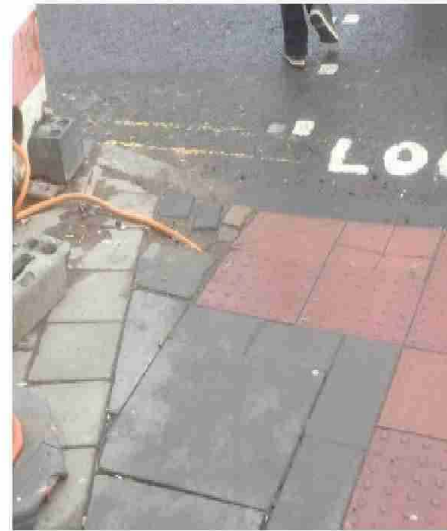
Cable on Surface at road crossing Trip Hazard – York Place
