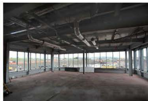
Gogar Depot Control Room
