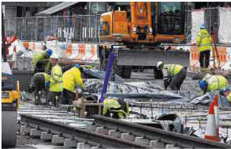
SLOW PROGRESS: An earlier dispute between the council-run company Tie and the group constructing the tram system led to work on Princes Street being suspended for a month last year.
