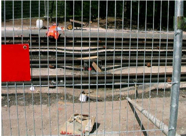
Figure C.11: Slab Beneath Rails Lowered Locally to Enable the Installation of Ducts and Pipes
