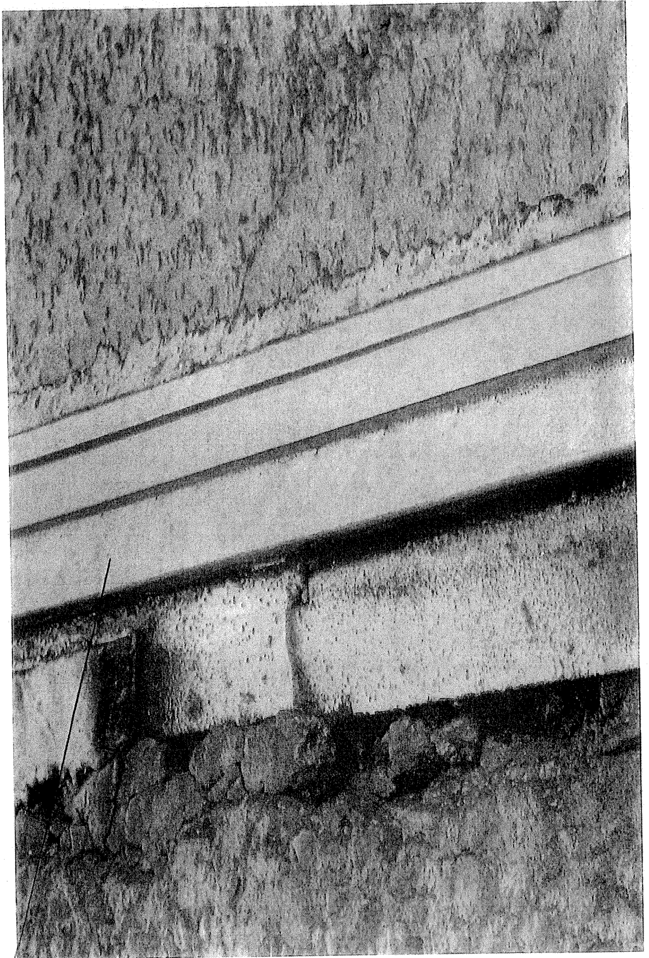
FAULT AFTER REMEDIATION - MOVEMENT IN THE OUTER CHAMBER & DEFORMATION
