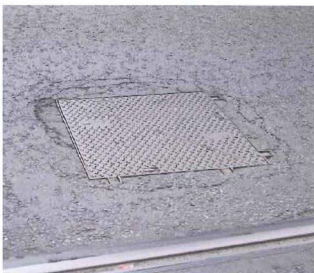
Poorly laid wearing course
