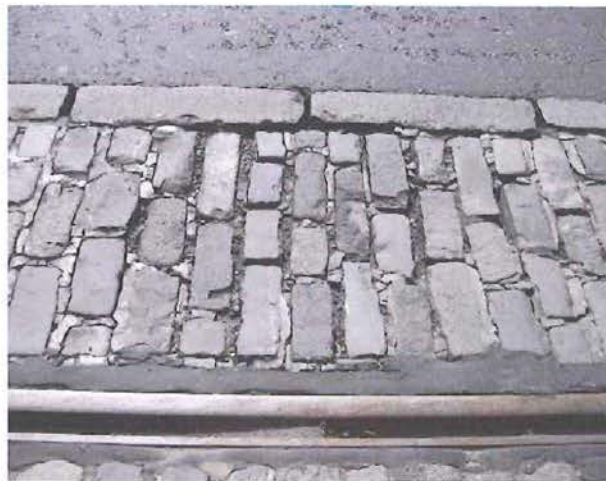
Failure of the grouting system is evident here....
