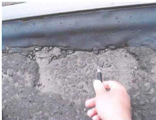
This photo clearly indicates how thin is the wearing course
