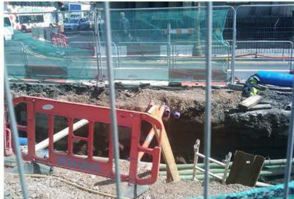
Photo showing shallow ducting
