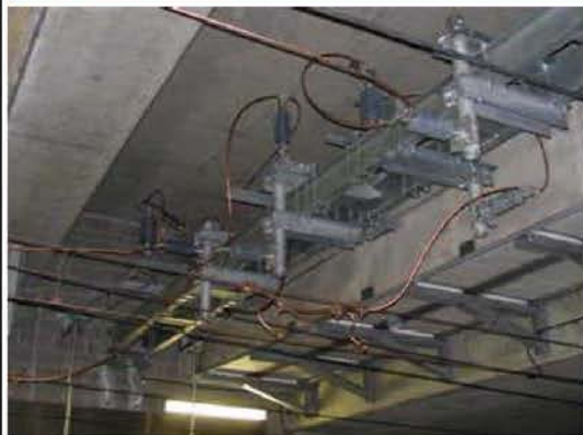
Completed Switches for SSI's
