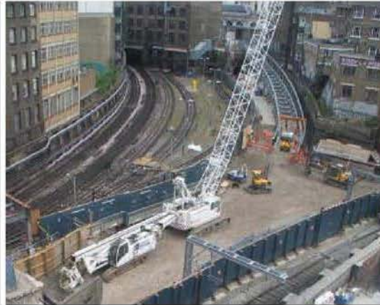
ITH east pile mat completed and piling rig/attendant crane tracked across RRAP
