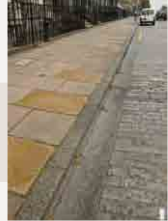
Kerb running parallel with boundary line
