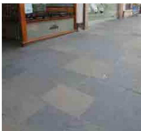
Odd size cuts on the inside of the footway
